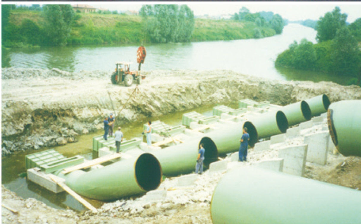
Drainage pumping station – Bresparola (RO)
