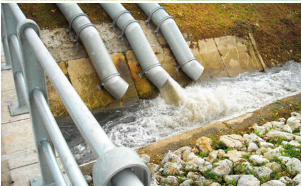
Drainage pumping station – Torri di Quartese (VI)
